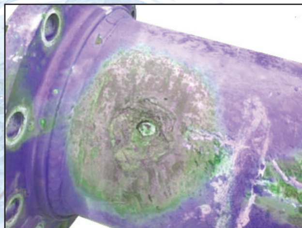
Corrosion of the vent hole area following permeation and no particular corrosion protection
